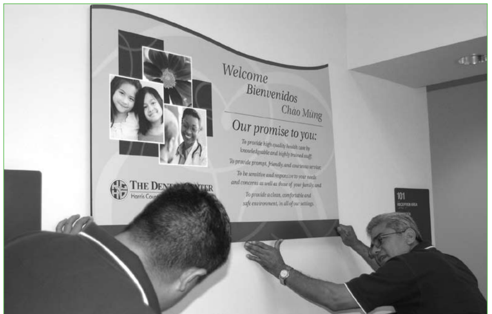
Workers install new signage in the lobby of HCHD’s Dental Center located at 5230 Griggs. The signs, which greet patients in three languages, are part of a district-wide initiative aimed at making visitors feel welcome.
